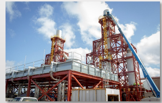
Schofield Barracks, Hawaii: 50 MW Biofuel/Multi-fuel Project operational since May 2018. Full "Islandable" energy capability expected for Schofield Barracks, Camp Kunia and Wheeler Army Airfield
